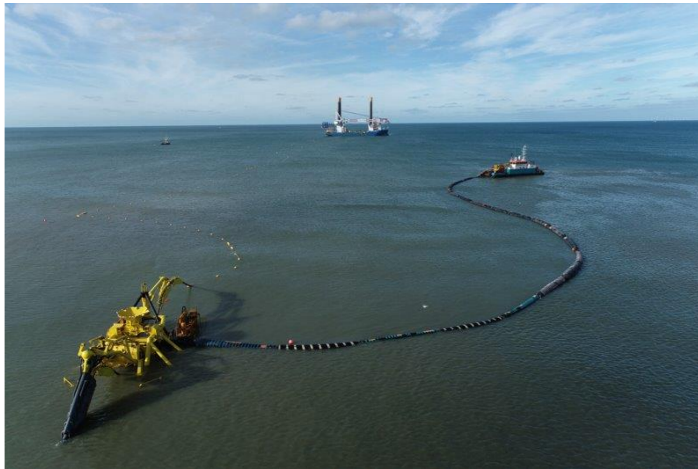
Figure 3.14: Example of shallow water trenching vehicle, with support vessels achieving subsea cable burial (photo courtesy of JDN contracting).
